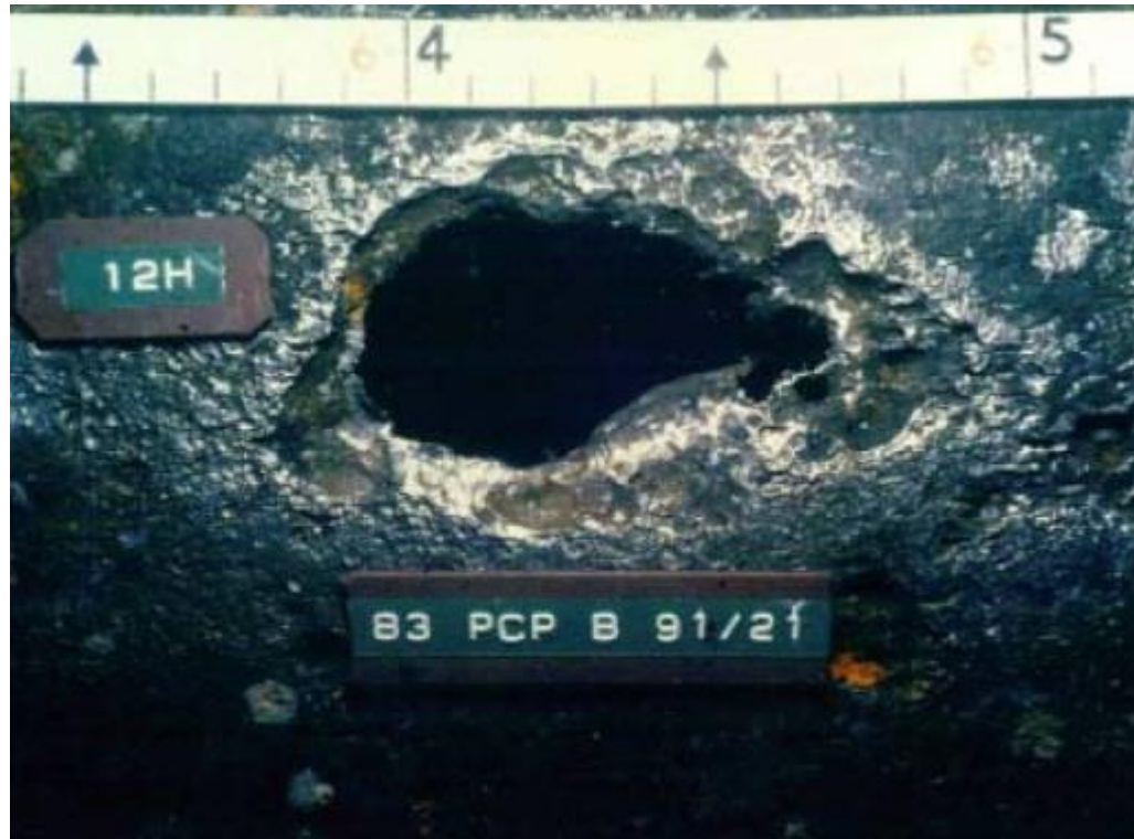
Corrosion of a bracing of jacket
